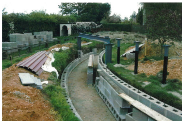
The tunnel walls starting to go up with the girder and supports for the over section. Old raised track in the background.
